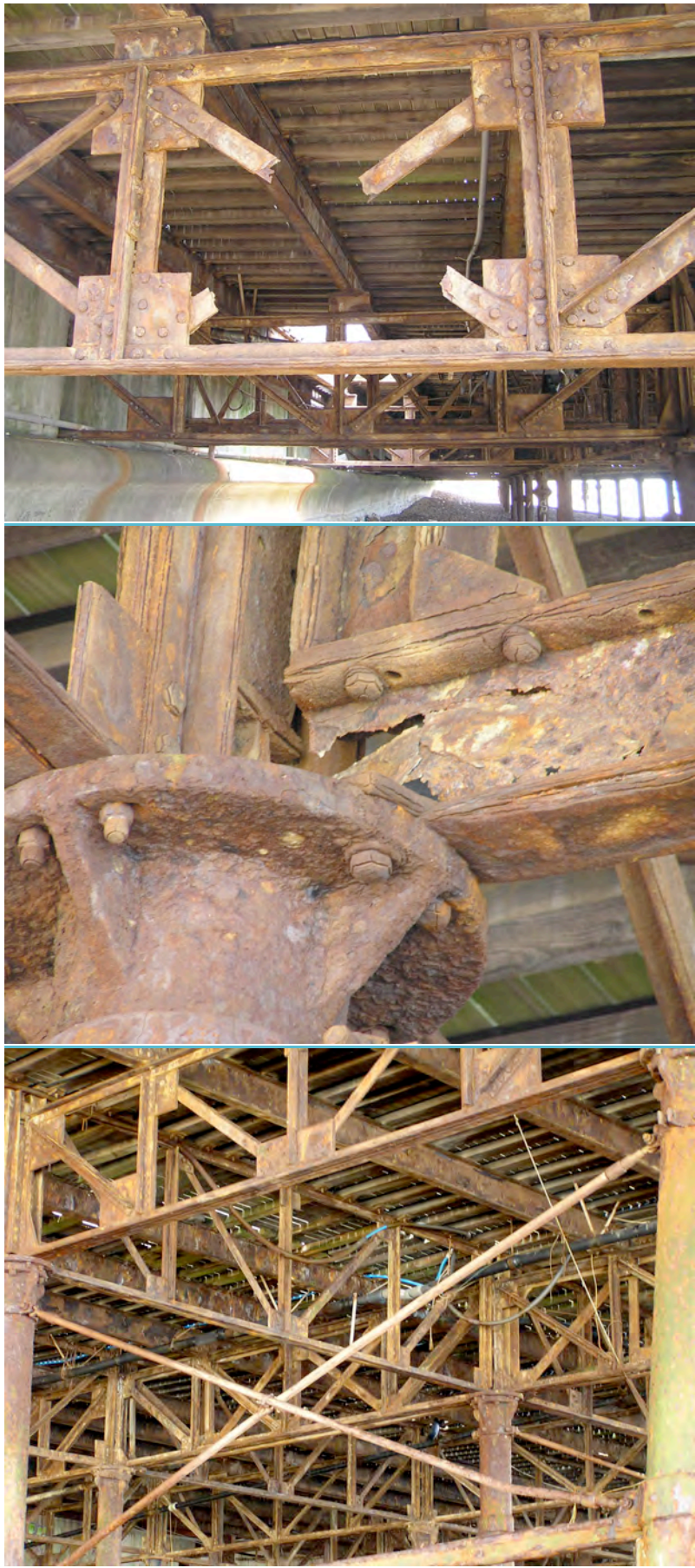
Corrosion and damage to the sub-structure
